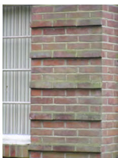
Picture 9.25 Projecting bricks
